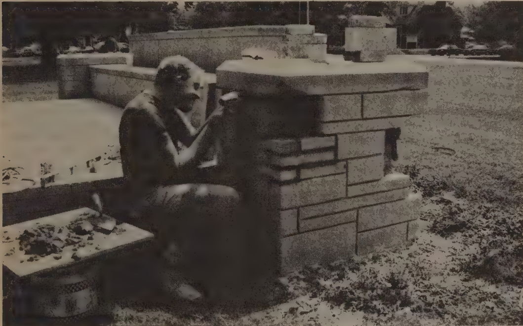
The UE sign located in front of the school received a face lift last Thursday when Ted Thompson, contracted outside help, resealed the loose stone and applied new mortar. (Photo by J.C. Gureghian)
